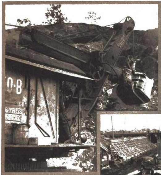
The Canadian National System Is Bucking the Breadline on a Big Scale. We See Here Just One of Its Many Construction Jobs—the Building of a Subway to Overcome the Level Crossing of C. N. R. Tracks over the Pembina Highway, a Motor Truck Road Connecting Winnipeg with Minneapolis and St. Paul via Emerson, Manitoba
